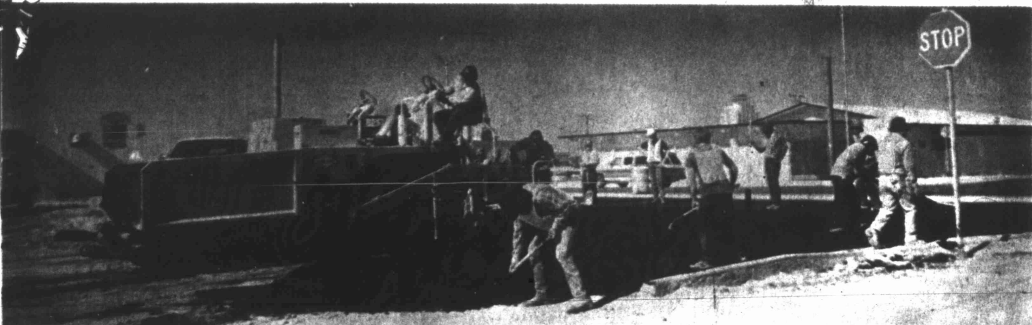
BIG SPRING — Workers lay asphalt on the road surface at the intersection of South Gregg and Sixth streets last week. A final inch-and-a-half layer of pavement will be applied beginning Monday, with officials asking motorists to avoid driving on the road throughout the week. For additional details, see the story on Page 8-B.
