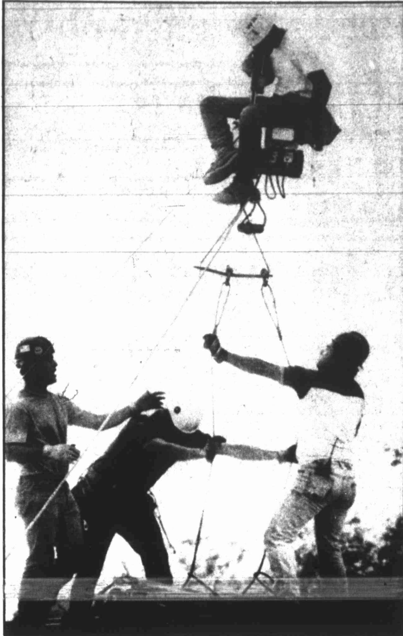
Easy does it SAN ANTONIO — Ironworker Henry Montez maneuvers a motor and cable with the help of his fellow workers while dismantling a scaffold on the Tower of the Americas at HemisFair Park, which was recently renovated.
