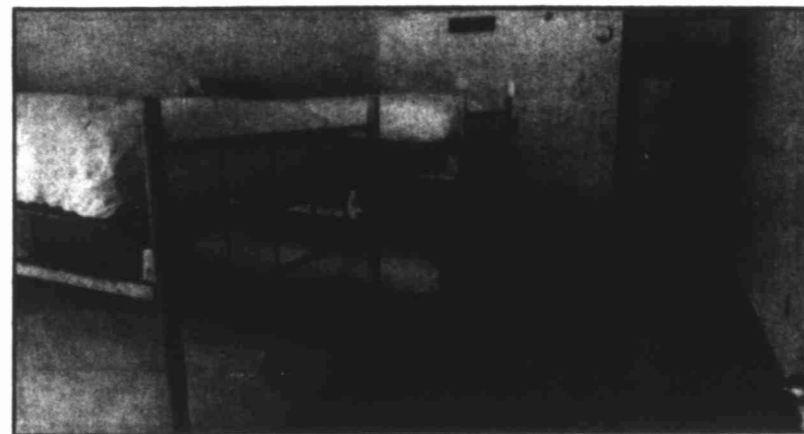
A set of beds in the prison will soon be used by some of the 250 inmates that will occupy the newly-renovated facility. The first contingent of 42 inmates arrived at the prison today and more are expected next week.
