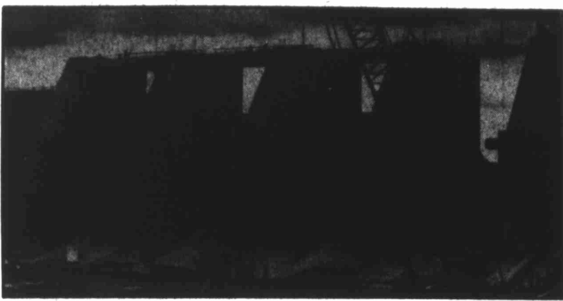
STACY DAM SITE — Construction continues on the Stacy Dam spillway, as three of the dam's six gates are already in place. Closure is expected in mid-November.
