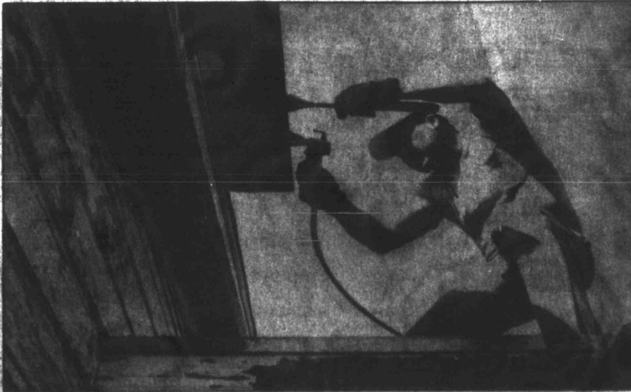
Simon Correa sprays a coat of primer on the overhang of a house at 1104 Mulberry. It was all a part of the work done by members of the
