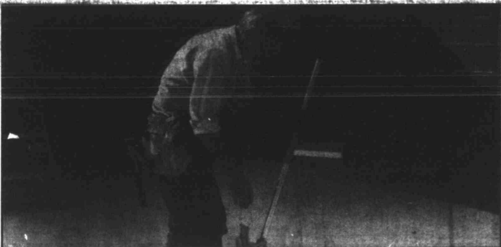
Carl Lawson bends conduit to install in what will be a classroom when construction is completed in 1990.
