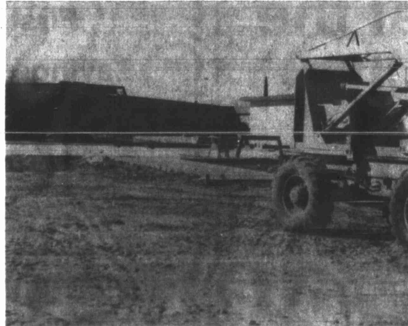
for the new Stanton Junior High gym. In center photo, a section of the finished gym foundation and a piece of equipment used to hold trusses in place while workers secure them are shown. The machinery, that
