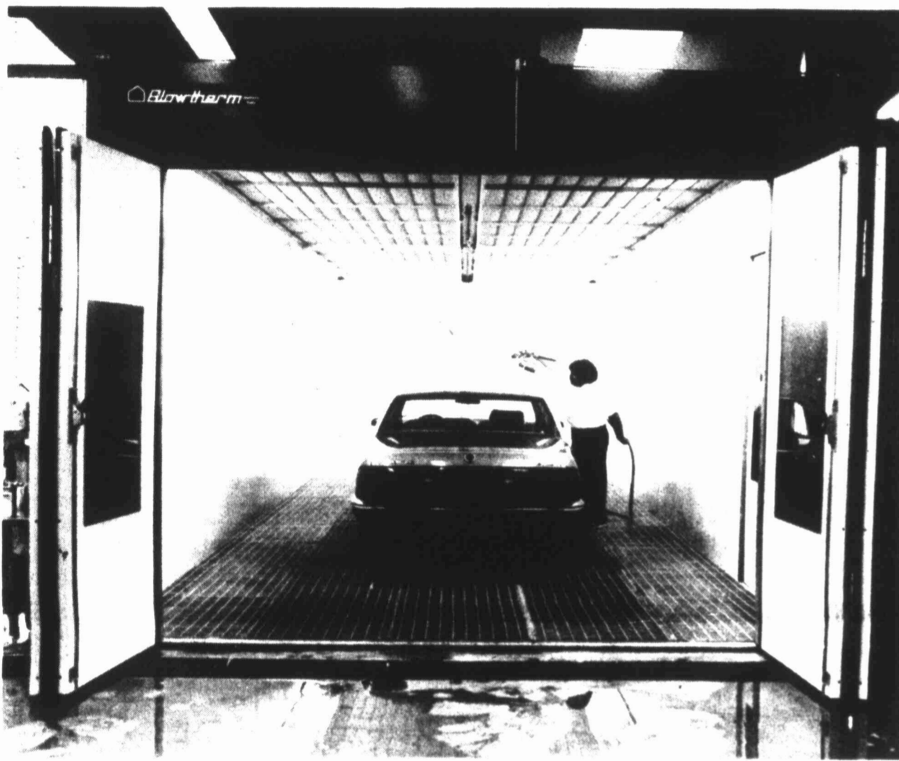
The new Blowtherm Ultra spraybooth oven produces the finest finish on automobiles this side of the factory. The facilities at Pat Gray Body Works underwent extensive alterations to accommodate the imported equipment. A factory-perfect paint job is made possible by perfectly controlled air, humidity and temperature.
