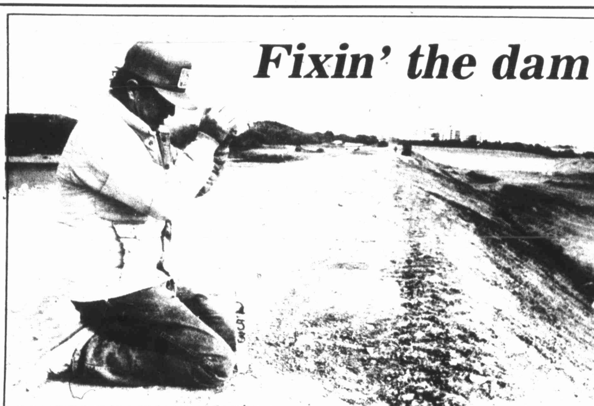
Farris Smith, an employee with Versatile Construction of Logan, N.M., hammers a stake in place as work at the Comanche Trail lake dam.
