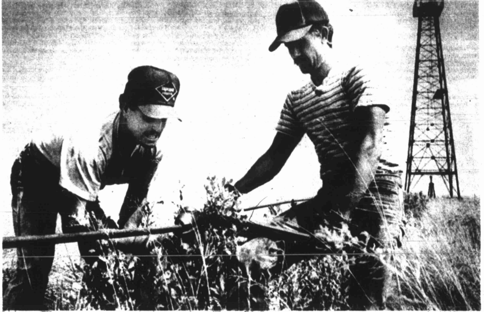
Salvaging KELLERVILLE — Roustabouts Jeff Pike, left, and Bobby Anderson salvage a pump cable.
