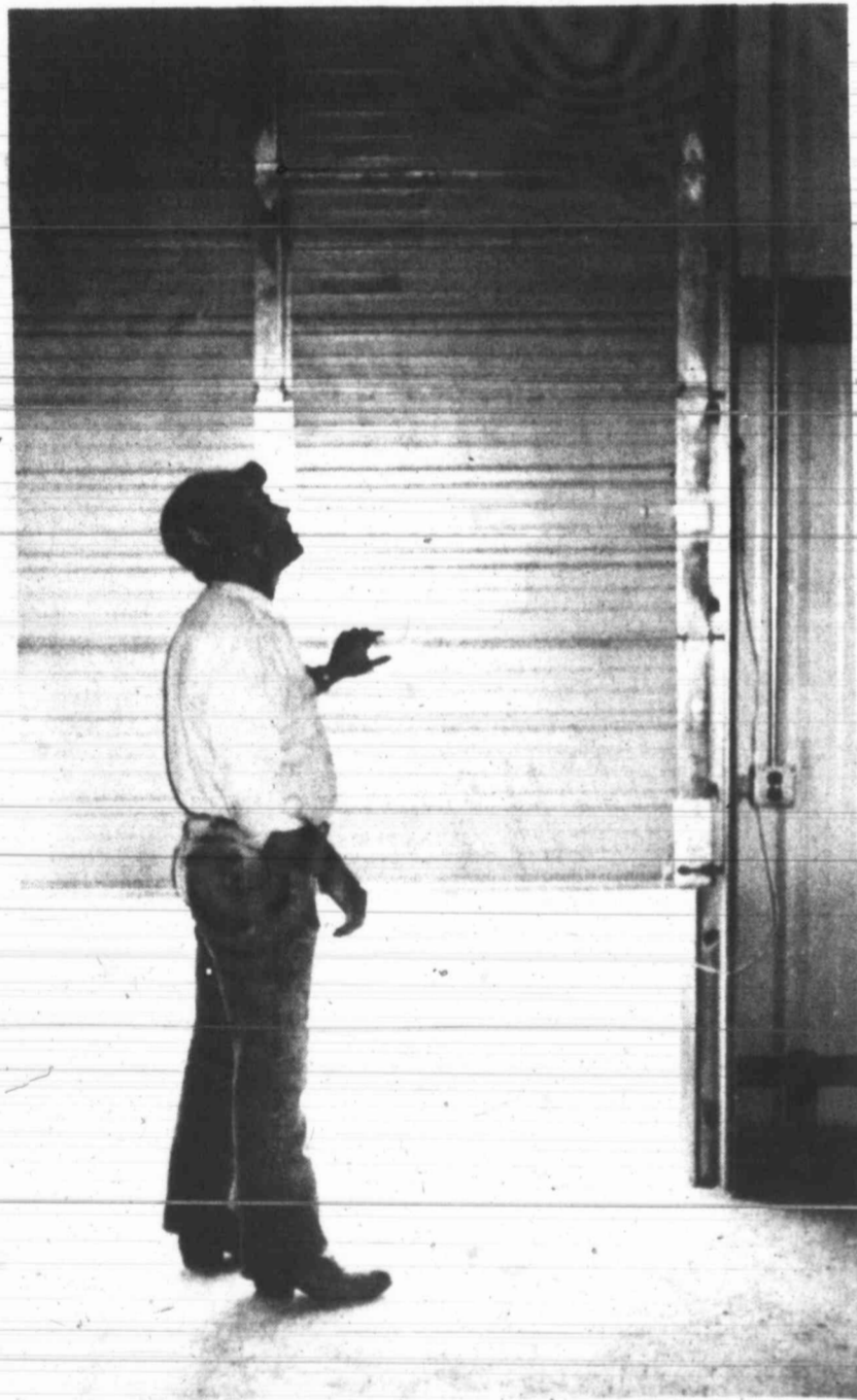
OVERHEAD DOORS — Reinert Welding & Steel Construction installs overhead doors for garages, storage buildings and commercial buildings. Ralph Reinert, owner, is checking the installation of a recent job.
