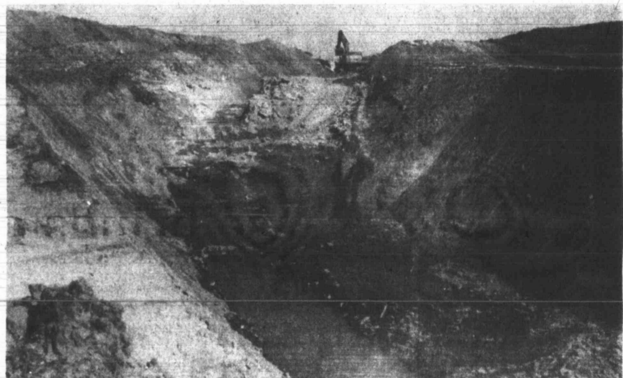
eventually be underwater when the dam is completed. At right is a scene of the construction work now underway.
