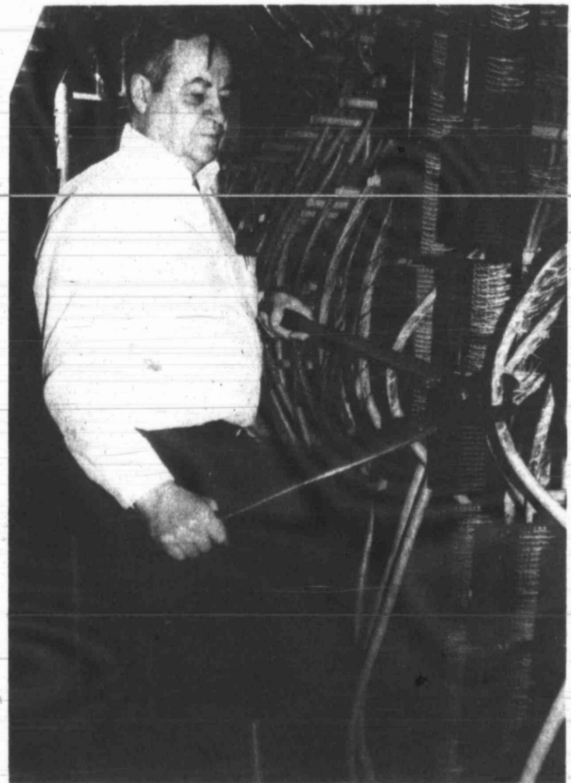
New system Jack Armstrong prepares to cut a telephone cable in the Southwestern Bell building on the corner of Eighth and Runnels, Friday afternoon. Armstrong, who helped install the old switching system in 1953, is retiring with it. The new switching system was activated midnight Friday. Local residents must now dial all seven digits.
