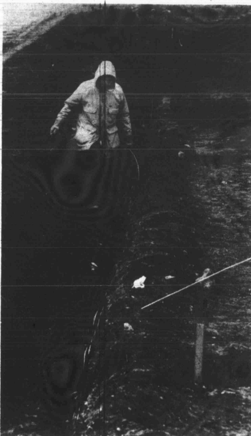
An unidentified city worker lays new lines to accompany the city golf course irrigation lines. The renovations were part of several efforts in the city, including swimming pool repairs and Comanche Park improvements.
