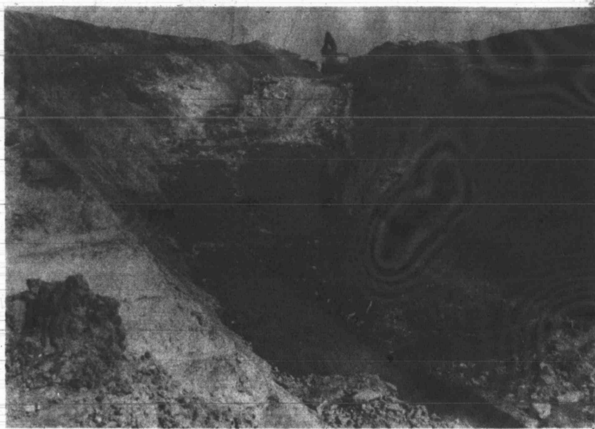
eventually be underwater when the dam is completed. At right is a scene of the construction work now underway.
