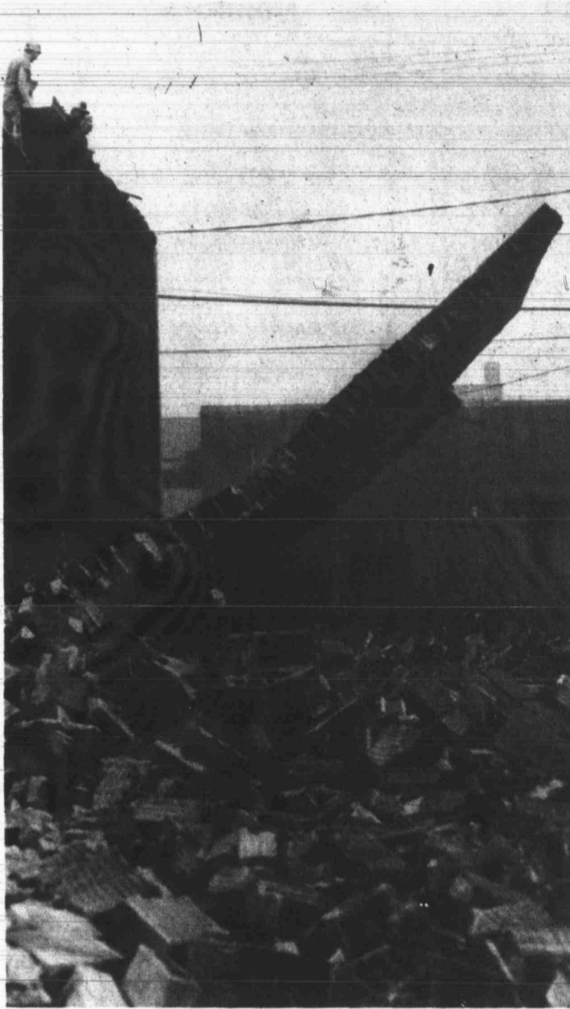
A wall adjacent to the downtown "pocket park" on Main Street tumbles into rubble at the beginning of renovation efforts in October.
