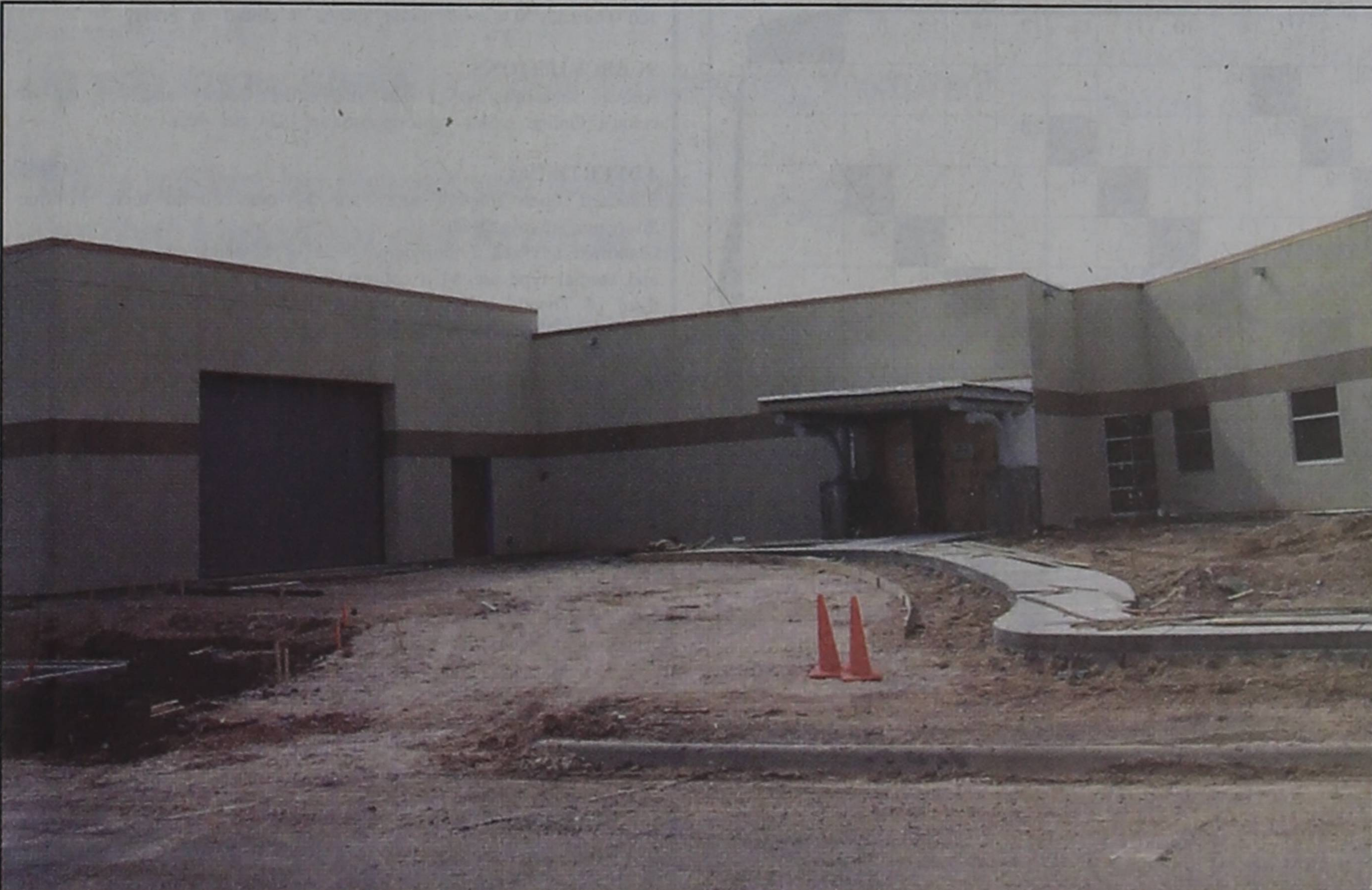
Construction continues on the new hospital. Workers have begun pouring the curbs and driveways on the 14 th Street side of the building. Much of the work has now moved inside. Officials hope for an opening in the summer.
