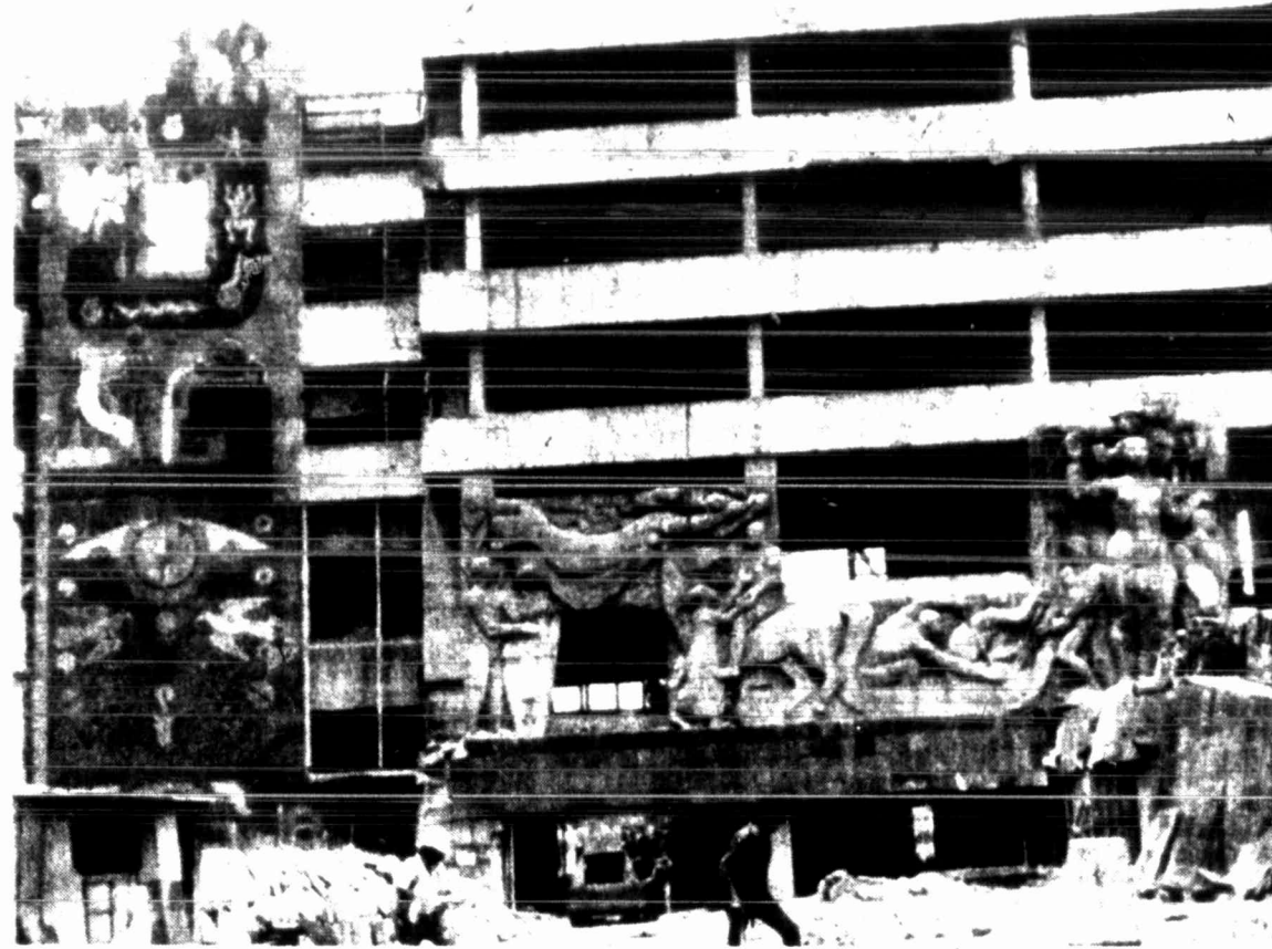
The lower floors of the Communications and Transportation Department's building in Mexico City were preserved to keep intact their murals. The upper floors were demolished, causing one of the most serious losses to the city's murals from the Sept. 19, 1985, earthquake.
