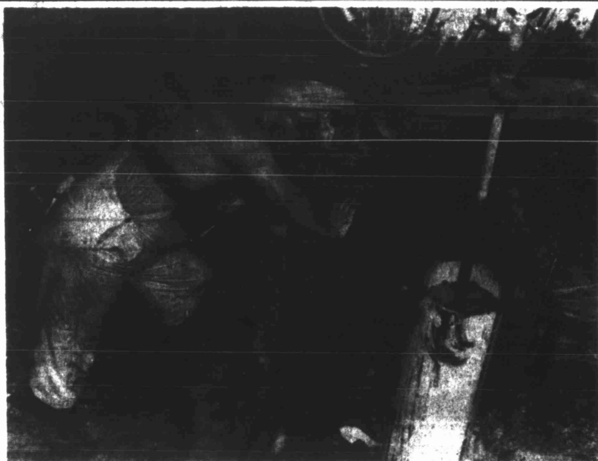
City employee Ronnie Whitley tightens bolts on a troublesome gate valve after attempts to de-pressurize it last night failed. Crews worked for more than three hours attempting to remedy the problem at the water plant that has hindered the city's ability to keep its reservoirs full. Crews today are looking for alternate ways to stem the pressure.
