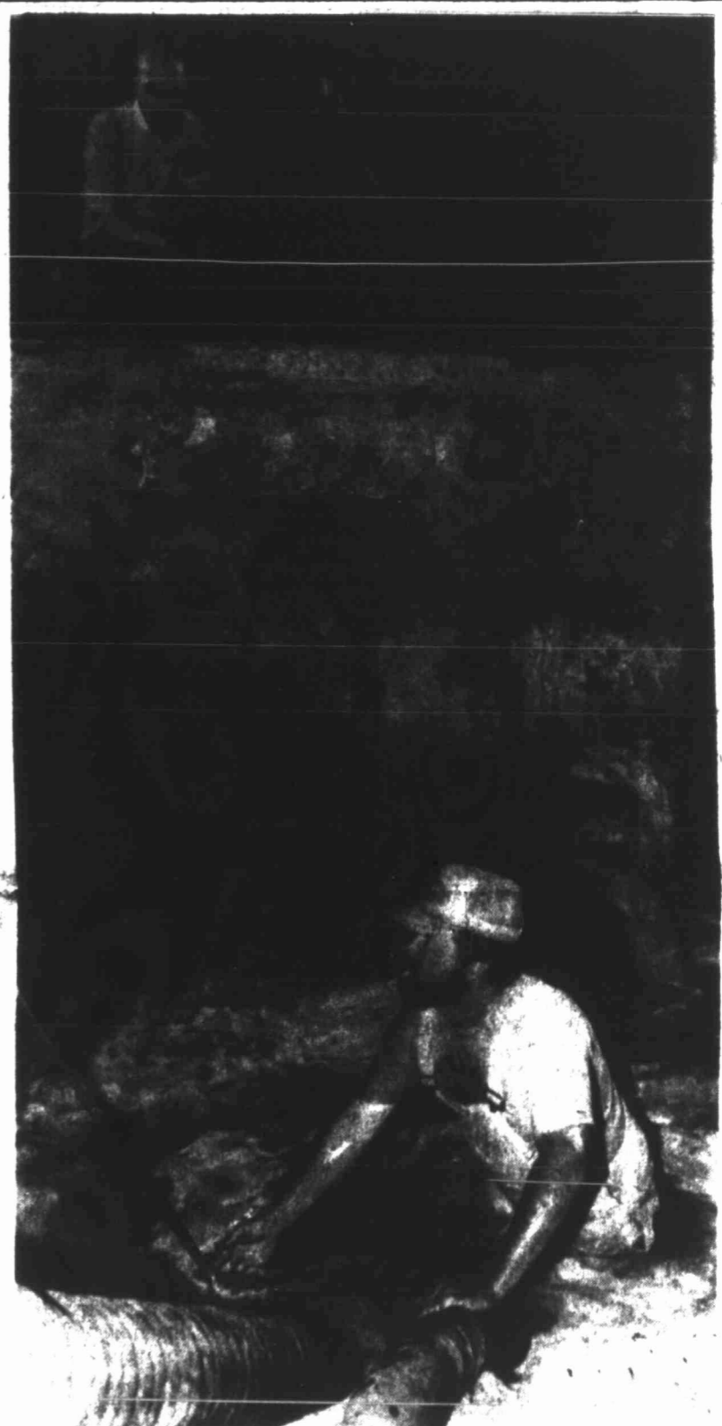
Ronnie Whitley is waist-deep in water as a suction pump hose becomes clogged with mud. Whitley was in the large hole helping to correct a problem with a malfunctioning valve in the city's water system.
