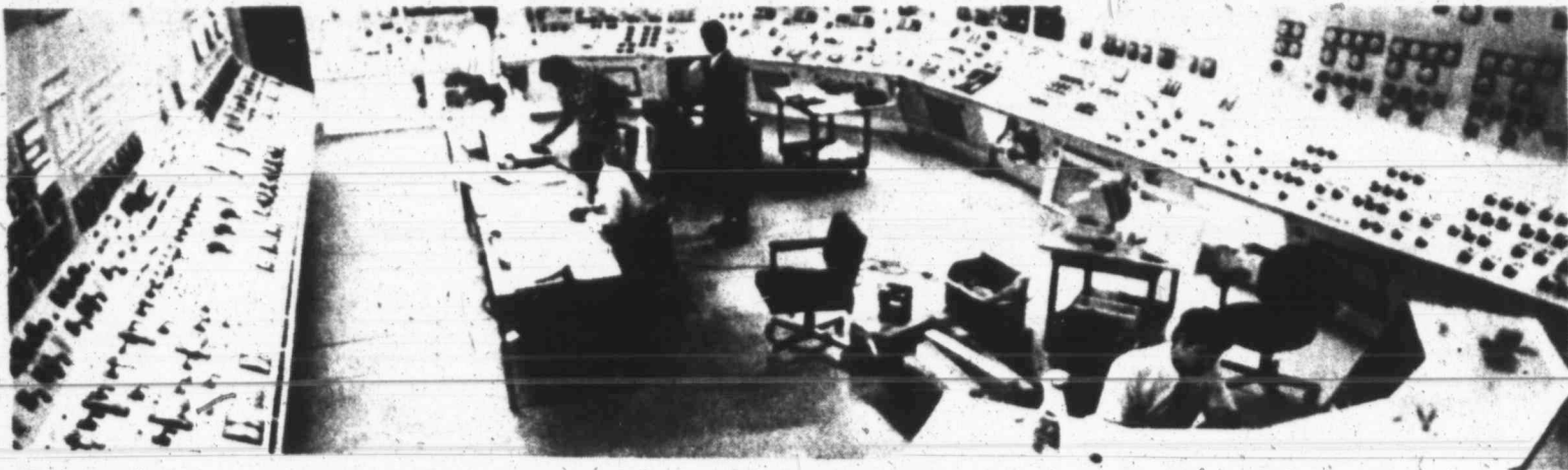
An $8 million control room at South Texas Nuclear Plant is used to train the people who will run the plant from day to day.
