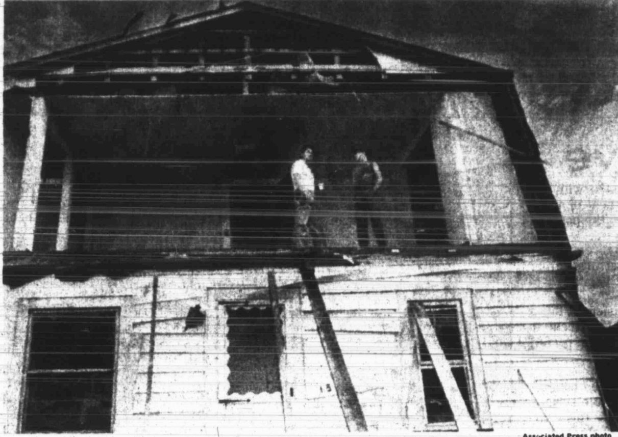
Robert Lewis and his son stand on the second-floor bedroom of their home in Niles, Ohio, Sunday surveying the damage done by a tornado that moved through the town Friday evening. Lewis stayed in the house waiting for the insurance adjuster to arrive.
