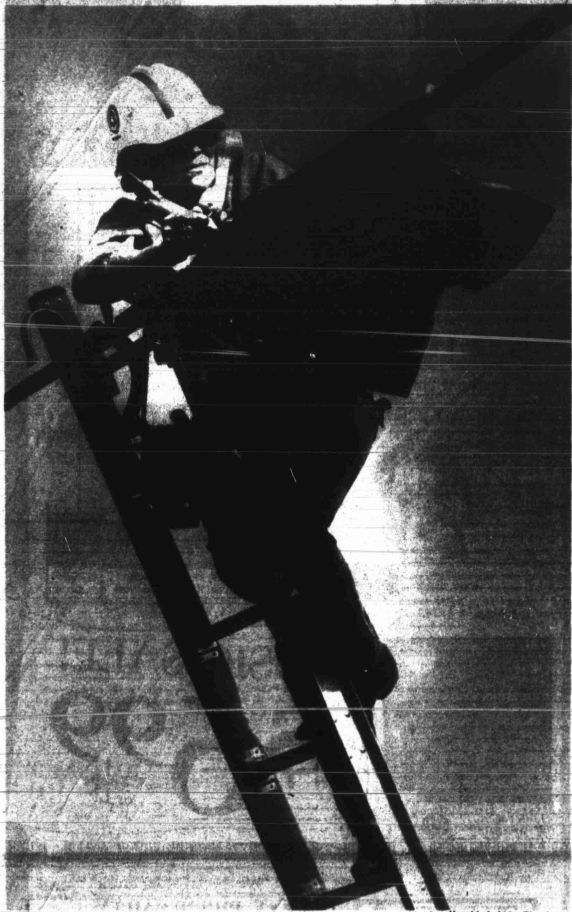
WORKING ON A CABLE — Paula Bayes, one of Southwestern Bell's cable repair technicians, prepares a 300-pair, paper-insulated telephone cable and listens for a tone on her handset. She is working on restoring service to local resident's telephone. Herald photo by Tim Appel
