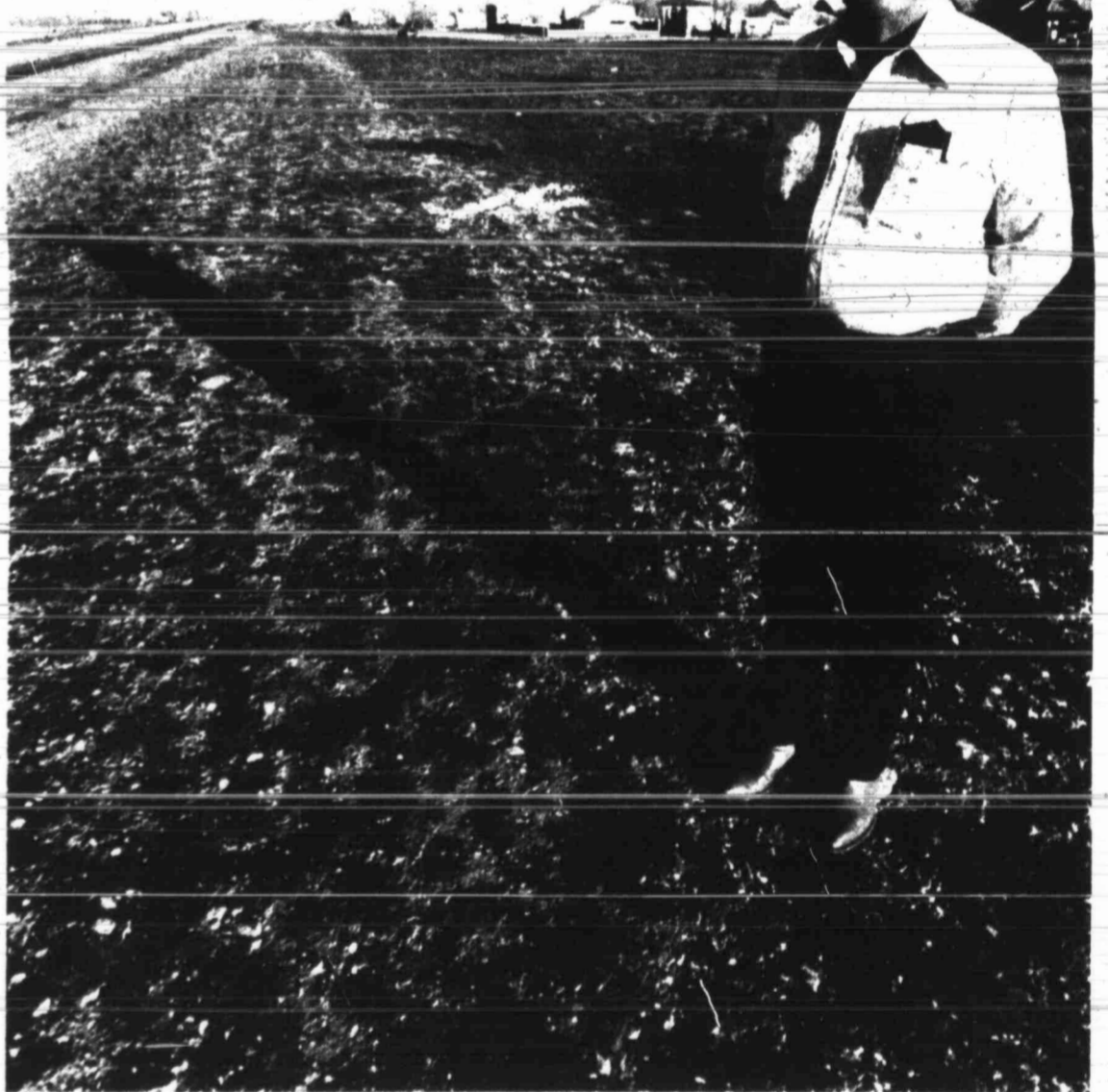
RAY HOLLIS stands near I-20 where he demolished a section of old homes to make way for Interstate.
