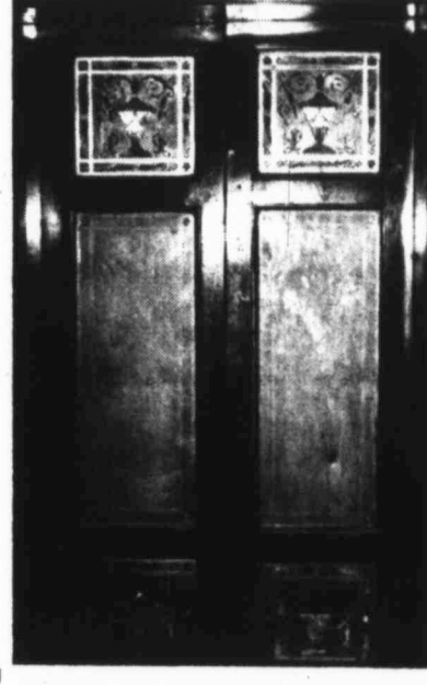
GOIN' UP — The gilded, first-floor elevator doors of the Hotel Settles stand scarred by years of neglect.
