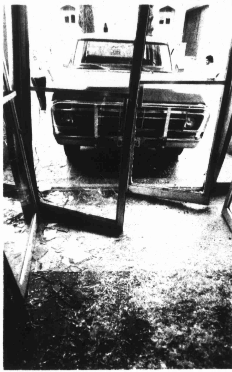
SHATTERED — A pickup truck, driven by a 35-year-old Big Spring man, rammed the front doors of the Big Spring Police Department on Fourth Street and shattered the glass doors. The man was immediately arrested on suspicion of driving while intoxicated and felony criminal mischief.
