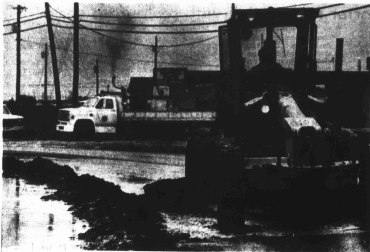
HOBBS FLOODING — Street crews in Hobbs, N.M., work quickly to build a dike along a street to hold back water being pumped from a neighborhood
