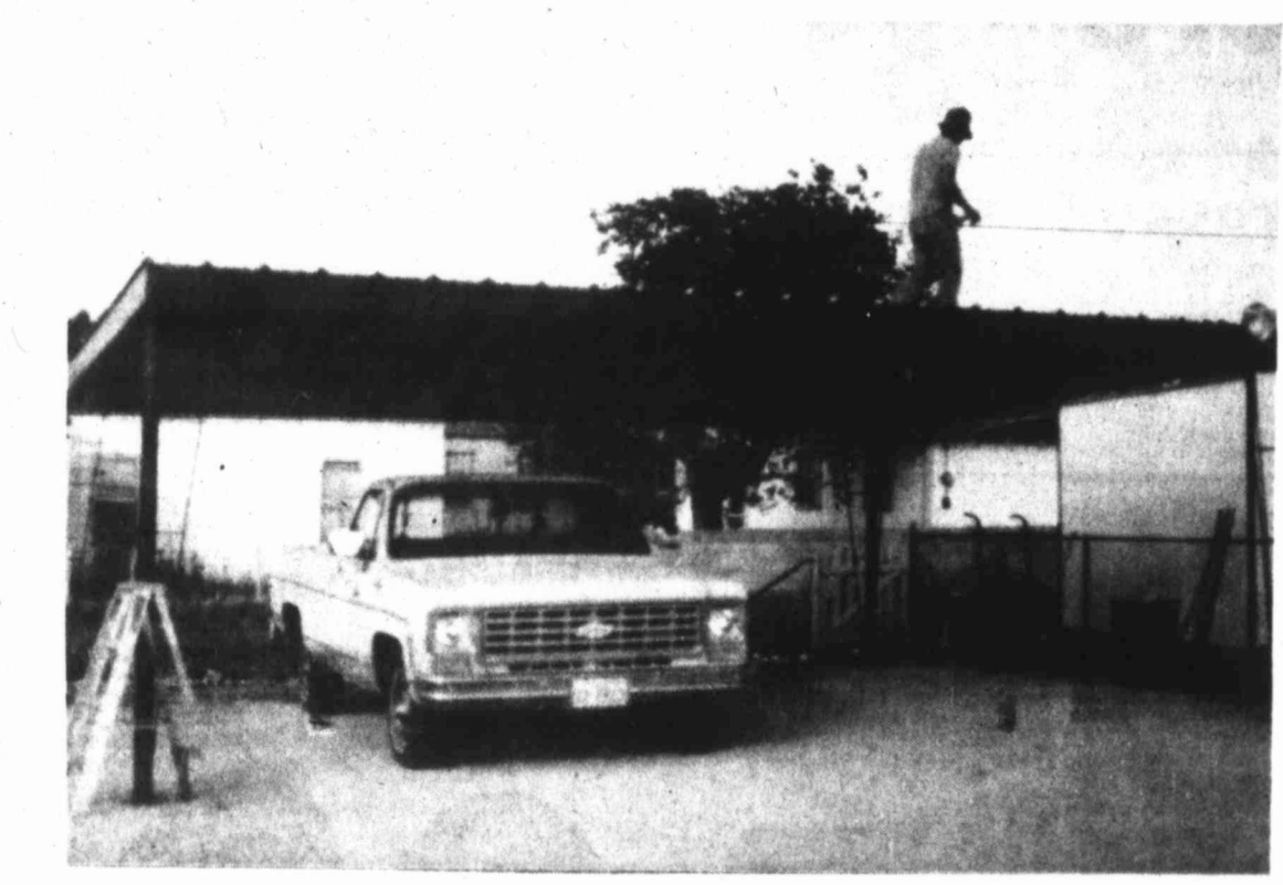
All-Weld Carports can be designed to fit any site and to accommodate any vehicle, including RV's.
