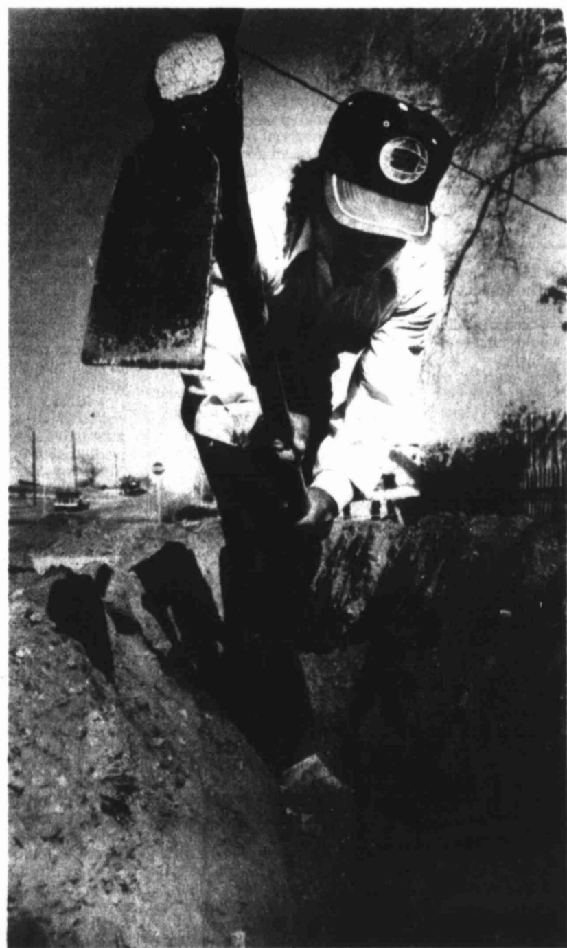
I CAN DIG IT — Albert De La Torre, an employee at Cline Construction, clears a trench along Eighth Street in order for his co-workers to be able to install a new telephone line.
