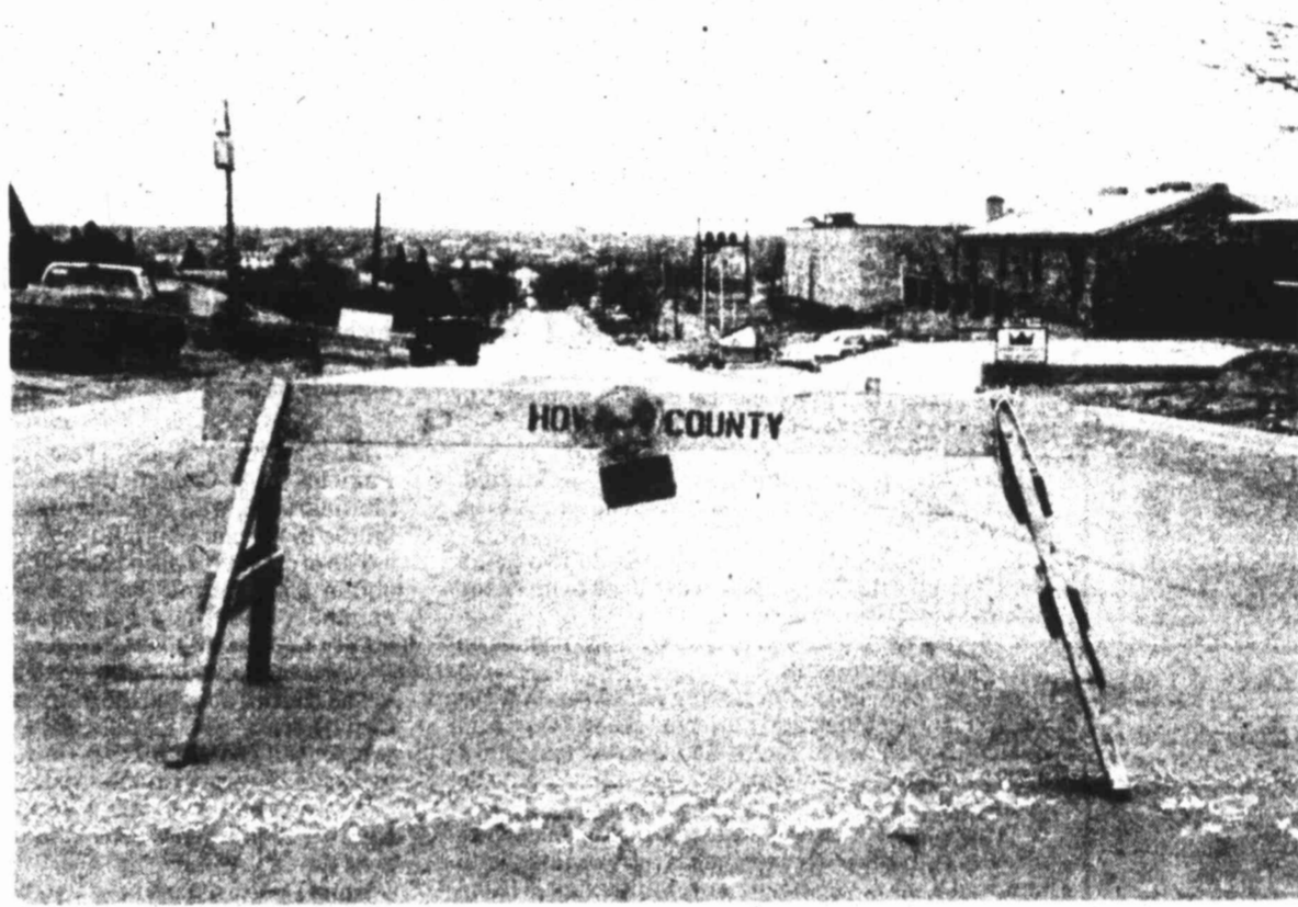
CLOSED FOR REPAIR — Several blocks of Lancaster road. The harsh weather of the past weeks has ruptured lines all over town and has kept crews scrambling to fix the breaks.
