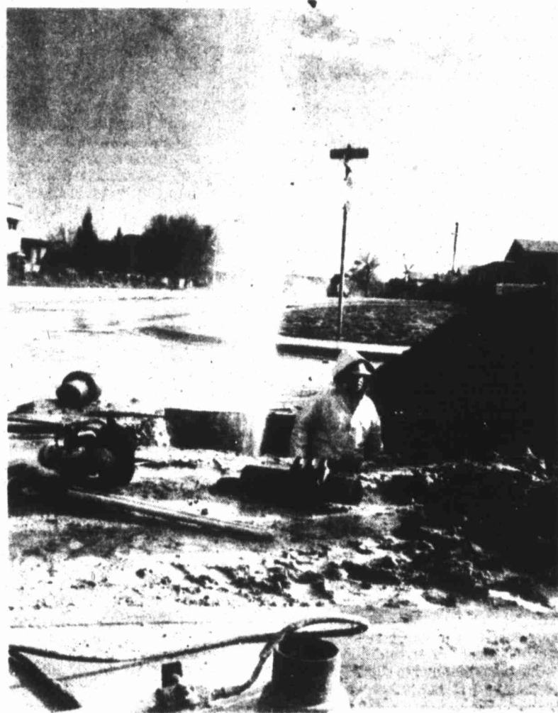
MAN-MADE RAIN — A Big Spring City employee seems perplexed as a water main at the intersection of Stadium and Birdwell is a bit troublesome to shut off after it broke and spewed water about 15 feet in the air. The city was able to effect repairs in a short while.
