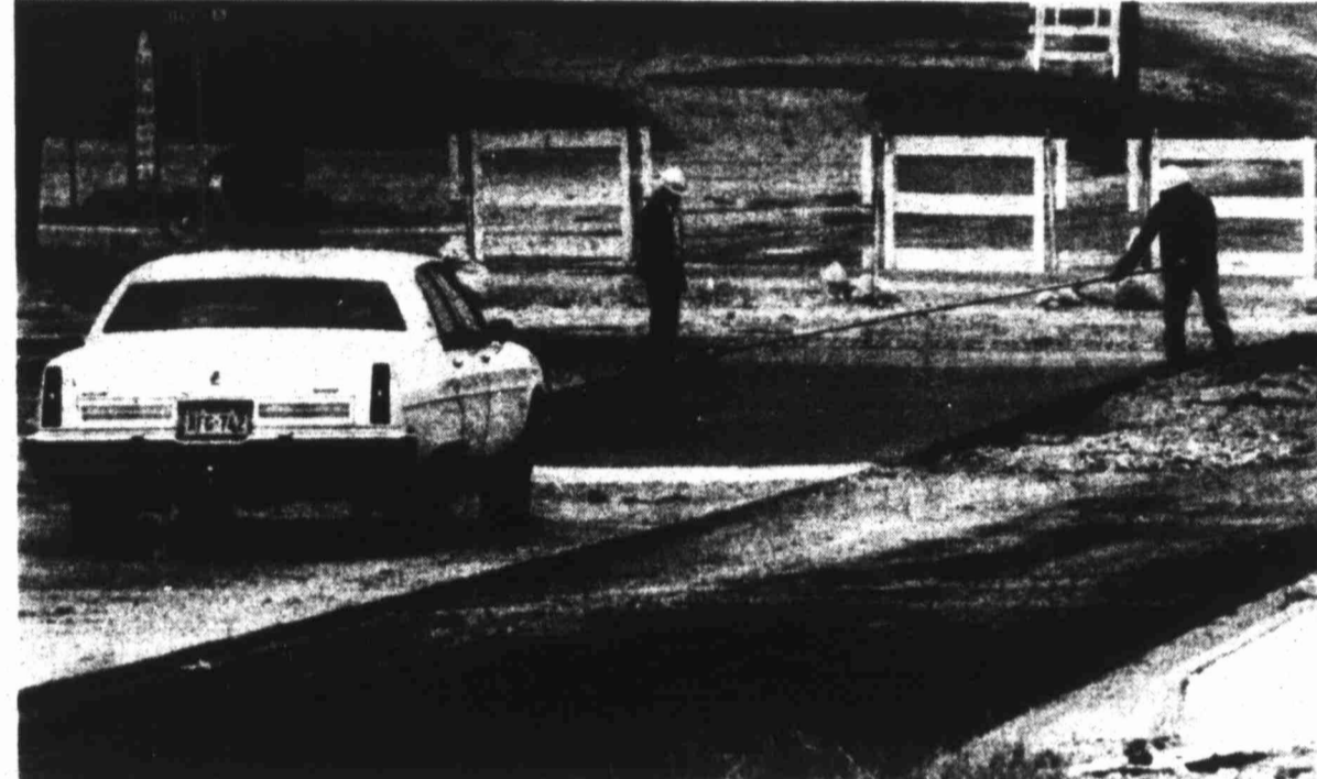
NOT YET, FOLKS — Employees of Price Construction Co. of Big Spring put the finishing touches on concrete laid Friday afternoon to correct a drainage problem.
