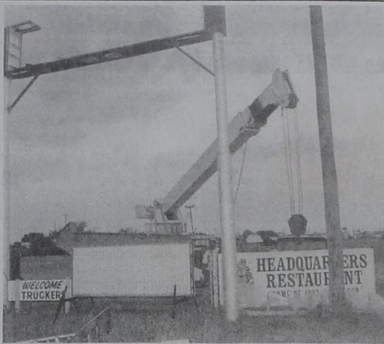
HERE'S YOUR SIGN.....Workmen prepare to hoist the new sign for Carl McInroe's Headquarters Restaurant to the top of the pole last week. The weather threatened to delay the sign installation, but workmen managed to beat the lightning and rain. (Ron Carr Photo)
