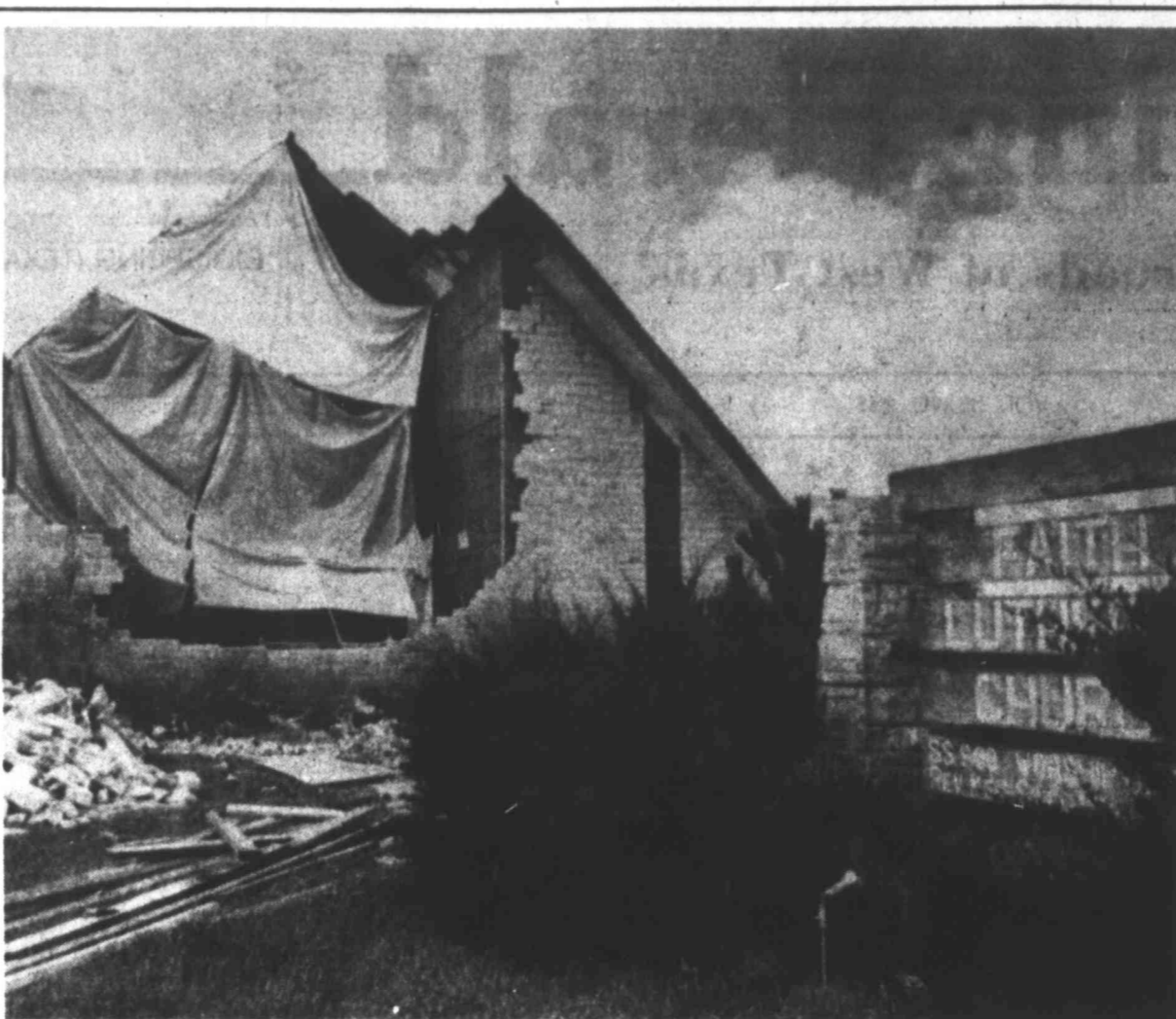
CHURCH HIT BY STORM — The Faith Lutheran Church in Sugarland has tarps draped over the front portion, to prevent further weather damage. The front of the church was ripped away when Hurricane Alicia passed through the area. The church congregation will continue to meet at a near-by Catholic church.
