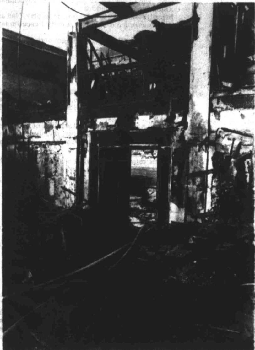
ROOF CAVED IN — This picture was taken on the inside of the building looking out onto Main. The roof collapsed at 1:30 a.m. and firemen brought the fire under control less than hour later, according to Fire Chief Jim Ryals.
