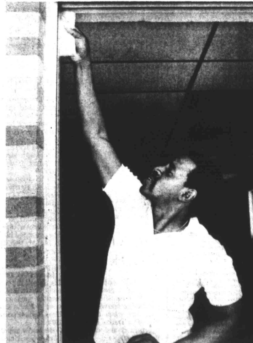
CLEANING UP THE RAINBOW — Archie Simpson stretches to clean the corner of a window at the Rainbow Project on West 13th Street. Simpson was one of six Big Spring Prison Camp inmates who spent Saturday putting the finishing touches on the shelter for abused and neglected children. An open house and reception are scheduled for next weekend.
