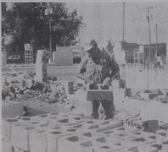
NO DIVING ALLOWED.... Friona city employee Chuck Teague joins co-workers in demolishing the city swimming pool. The city is furnishing the manpower for the demolition as a part of their matching funds grant. (Ron Carr Photo)
