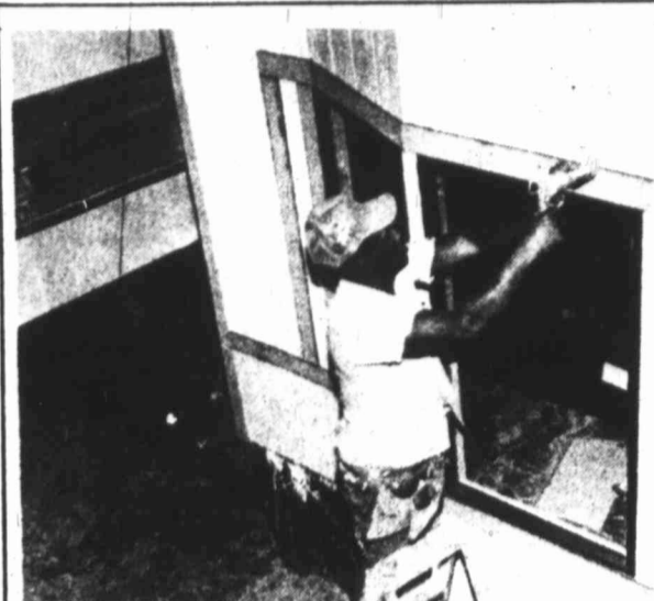
FINISHING TOUCHES — A worker at Cameo Energy Homes caulks a window on the assembly line of the Big Spring company. The company turns out about 2½ completed homes a day. According to reports, the manufactured-housing company did about $12 million worth of wholesale business last year.
