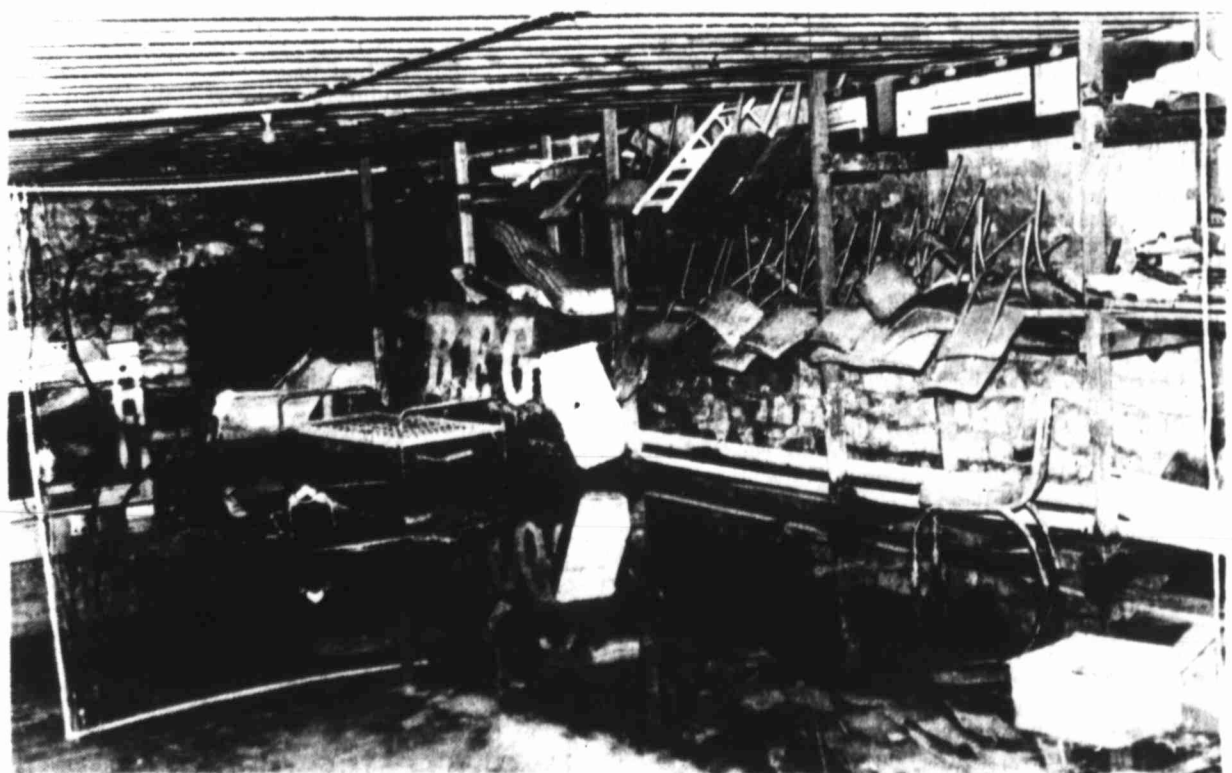
FLOODED BASEMENT — Briney subterranean water seeps into many basements in the flat area of downtown Big Spring, such as this one under the Atkins' family furniture store on the 100 block of Main.
