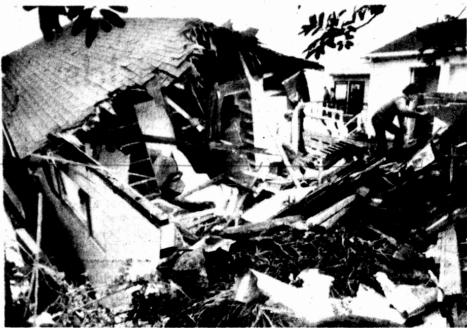
FALLING APART — Workers leave the wreckage of tennis star Billie Jean King's Malibu Beach home Wednesday after high surf and pounding waves slammed the home into an adjacent house. Workers later had to demolish the house before the debris was washed downshore to batter other seaside homes.
