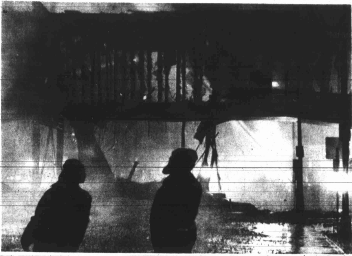
SKYWAY DAMAGED — Two firefighters gaze up at the Northwestern Bank Building. The walkway in the background shows the damage sustained by the fire.
