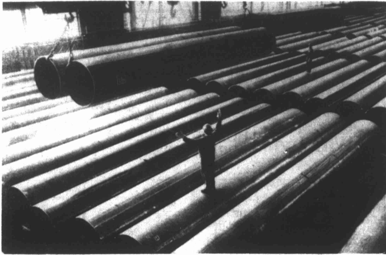
ON WITH THE PIPELINE — A Soviet worker directs crane handling sections for the Soviet natural gas pipeline. Released by the Soviet agency Sovfoto, the photo
