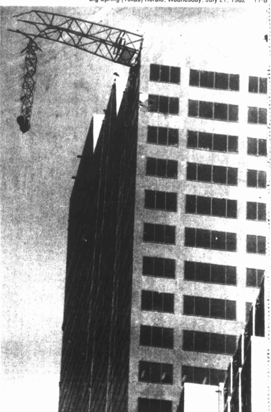
DANGLING OVER MIDDTOWN — Part of a crane atop the Continental Illinois Center dangles precariously about 60 stories above a New York street today. The crane fell onto its side sending debris crashing down to the street, killing one person and injuring at least three others.
