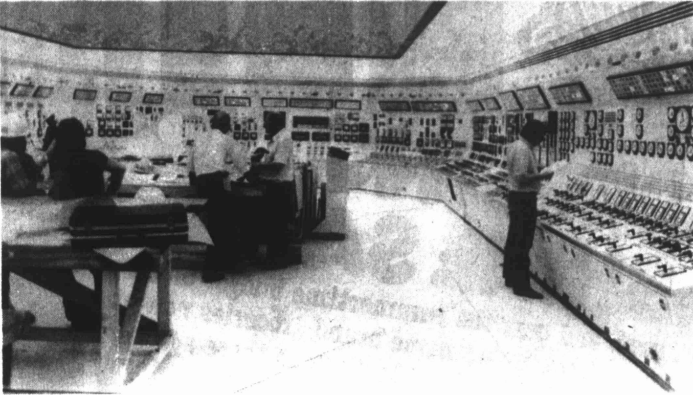
CONTROL ROOM — Part of the variety of switches and dials in the number one reactor's control room is shown, along with several workers. When the plant is operational, one controller will oversee the operation from this room.
