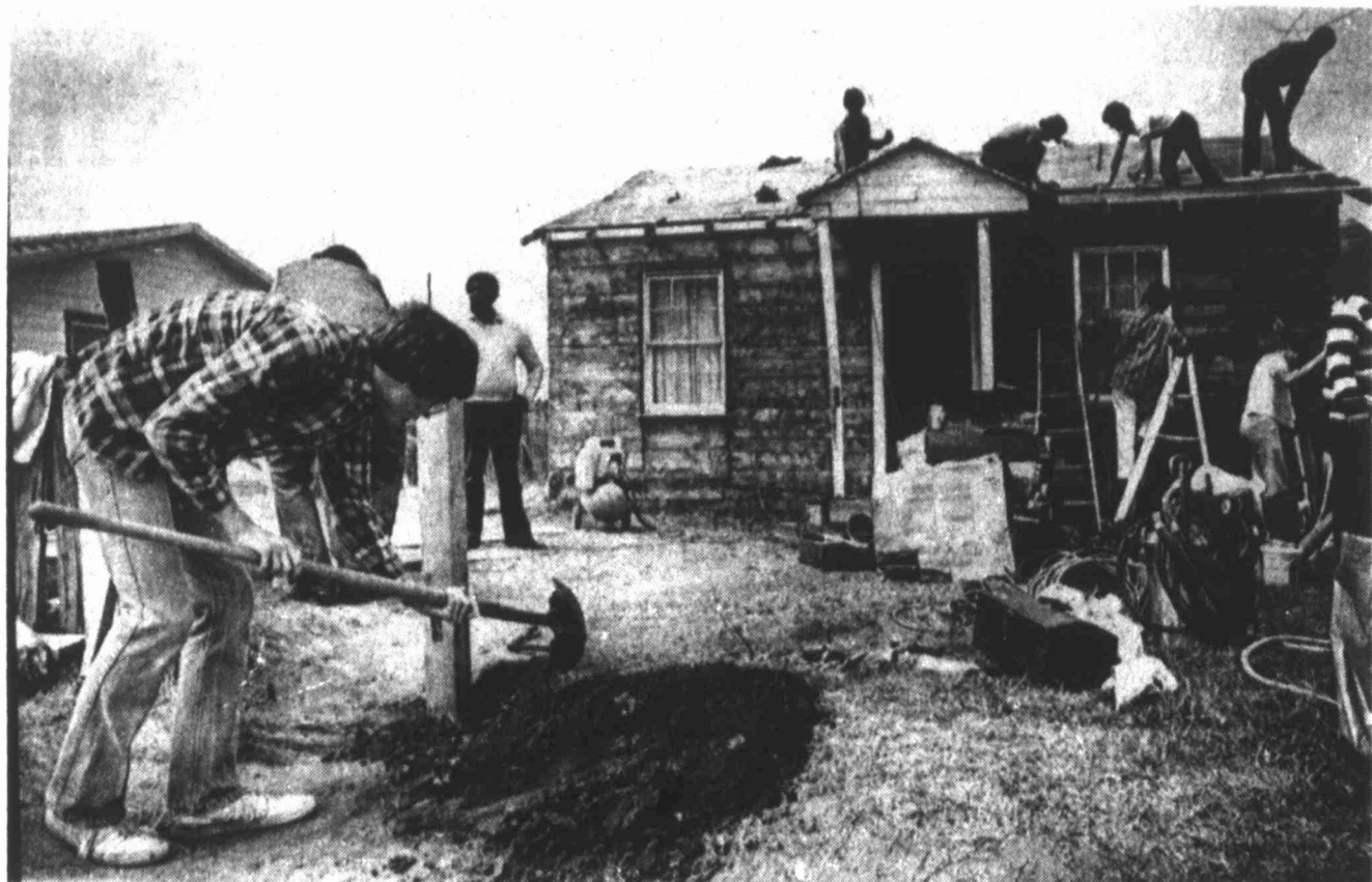
CHRISTMAS IN APRIL — Hundreds of workers decended on 144 houses that needed work ranging from roofs to floors in a flurry of activities that is the work day of the national famous Christmas in April project held
