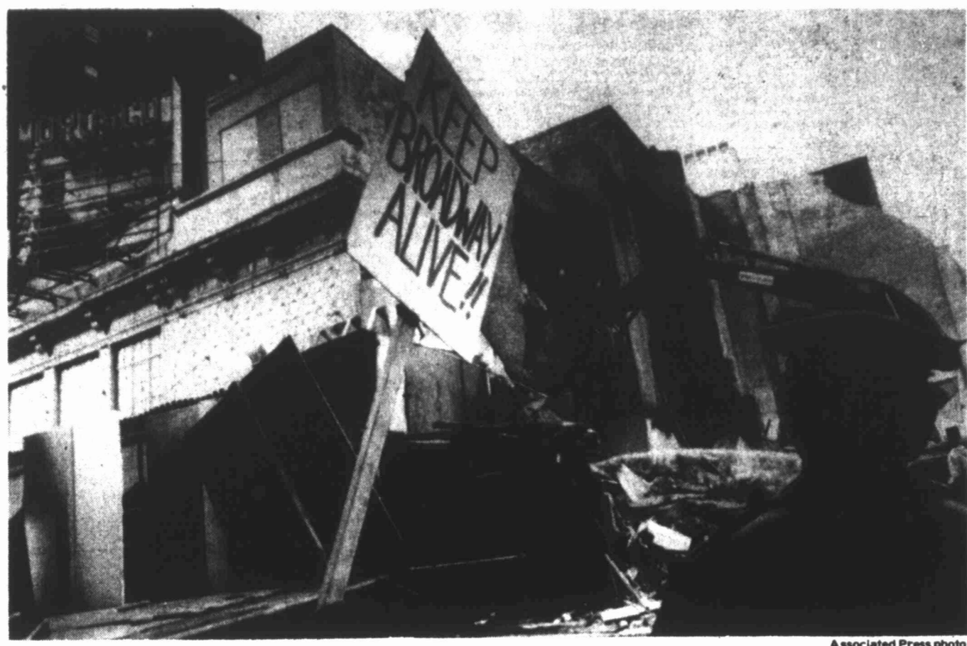
MOROSCO DEMOLITION — Policeman watches the wrecking arm bring down the side wall of the Morosco Theatre in midtown Manhattan Monday, despite public protest exemplified by the picket sign in foreground.
