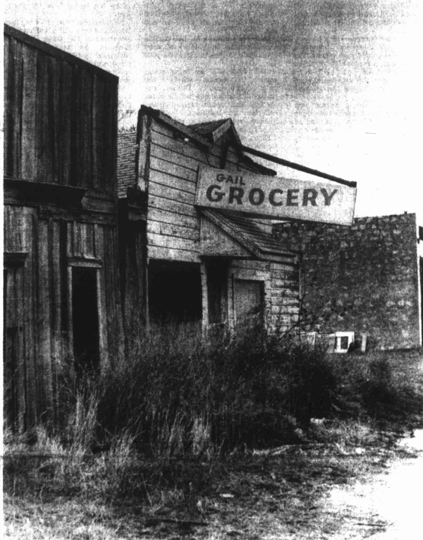
SAW BETTER DAYS—The old Gail Grocery on Highway 180 opposite the Borden County Courthouse obviously has seen better days. It closed about five years ago when it "just didn't seem to be a success," according to a county
