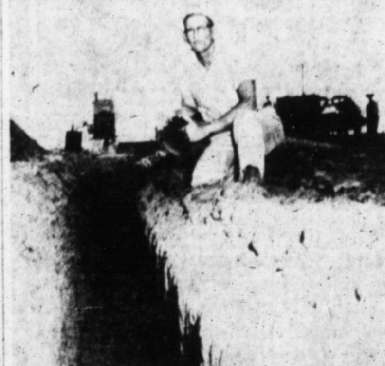
NEW SPRINKLER SYSTEM — James Thurman, who farms 3 miles southeast of here, inspects some of the irrigation pipe that is being installed underground on his farm. Some 4,275 feet of pipe will go into the system. (NEWSfoto)
