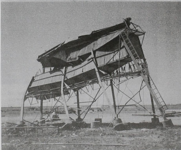
MONSTER FROM OUTERSPACE?-- The burr hopper on the old Co-op Gin property was being used for storage by Friona Wheat Growers Fertilizer plant. The tornado left it in a hazardous condition and plans are being made to tear it down.
