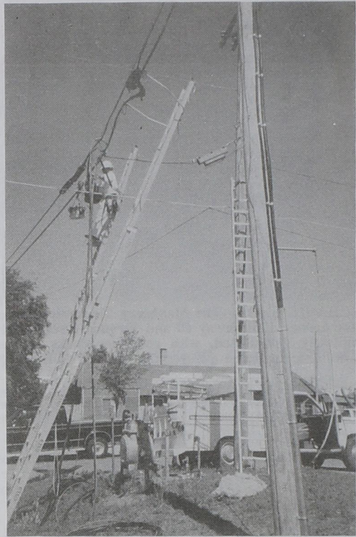
POLE PEOPLE --Everywhere one looked last week, there were people up on poles working to restore services to the homes and businesses in Friona.
