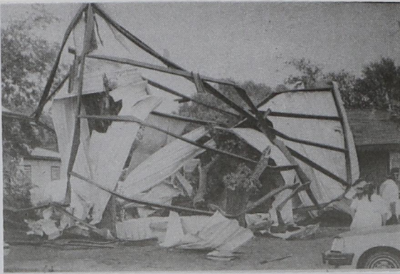
ROOF DAMAGES HOME-- The roof of the ambulance bay at the Fire Station blew over onto the home of the Mark Rodriguez family on Washington Street.
