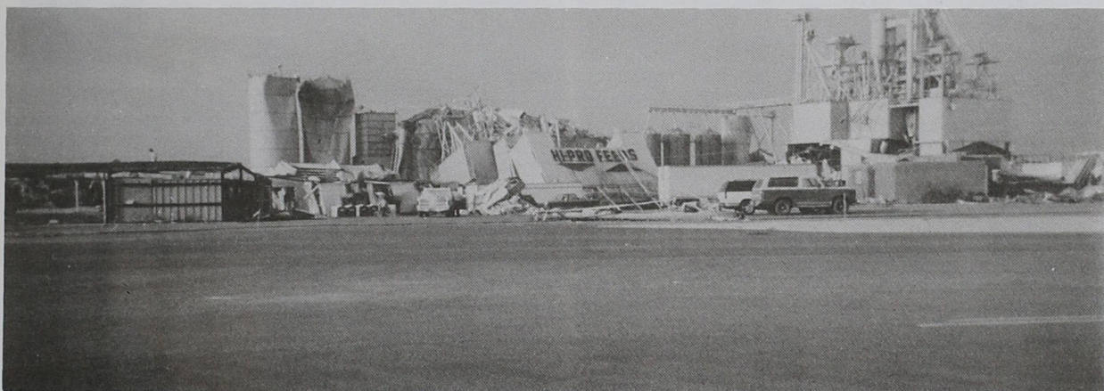
Hi-Pro Feeds, on the eastern edge of Friona, was in the direct path of the tornado.
