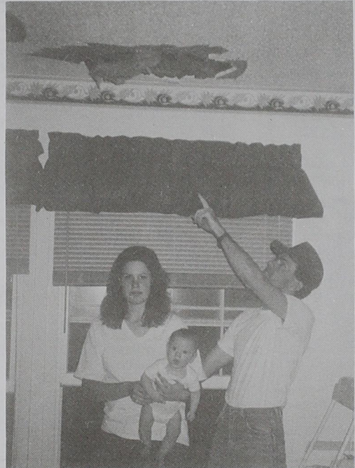
HOLE IN CEILING --Jerry Shields points to a hole in the ceiling and roof of his house where a concrete block came through during the tornado, landing in the baby's stroller. Jerry, wife Heather and baby J.W. were all in the basement. The block was thrown from the Stanberry building on the highway.
