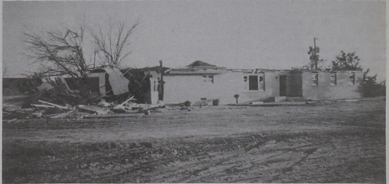
HOME OF BOB & LYDIA WYLY, ONE MILE NORTH OF CEMETERY, WAS DEMOLISHED
