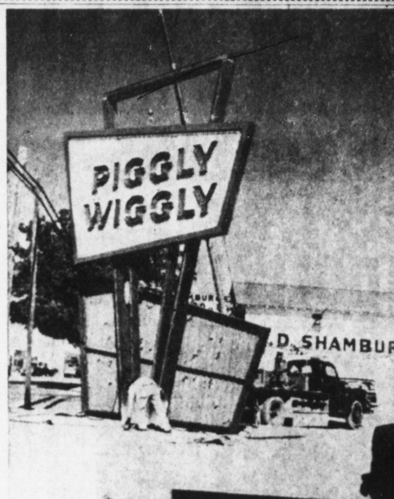
NEW SIGN — Workmen this week erected a new sign at Piggly Wiggly Super Market, replacing one destroyed by high gales last March. An estimated 32 yards of concrete went into the base of the sign. The three-color pattern consists of red letters on a yellow background and a green border. (NEWSfoto)
