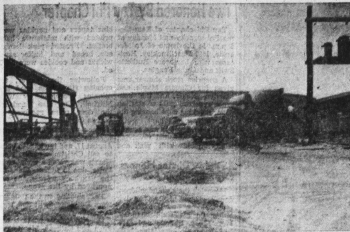
NEARS COMPLETION — Construction crews this week. The one million gallon water storage tank is in the center and portions of the water pumping station south of Coleman Park pumping set-up is on both sides of the picture.
