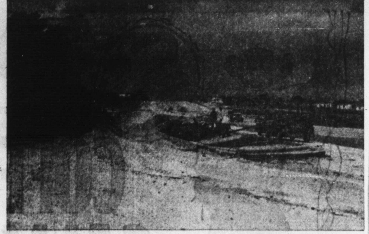
FOR NAUGHT — Highway construction crews attempted to complete masonry on this section of Highway 51 before clouds dumped their water early this week. The attempt was for naught, however, as the deluge flooded the by-pass road at left. (Staff Photo)
