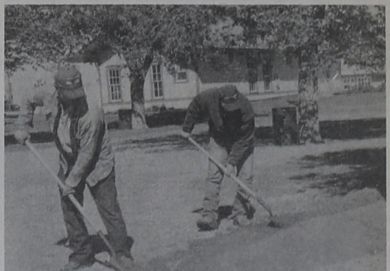
NEW SYSTEM --City workers were busy this week installing a new sprinkler system in the City Park.
