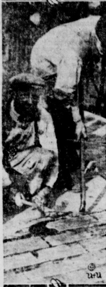
Rubber sidewalks and roadway are being laid on the north leaf of the Michigan avenue link bridge in Chicago. They are claimed to be "skid, wear and vibration proof."
